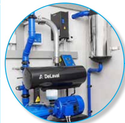
Vacuum system with DeLaval NFO
